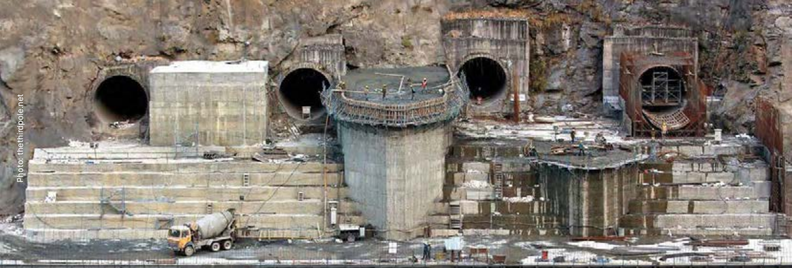
Construction work in December 2017 on one of the Punatsangchhu hydropower plant projects. The two power plants, the largest to be built in Bhutan, were supposed to be completed by 2020, but have been significantly delayed and caused additional costs.
